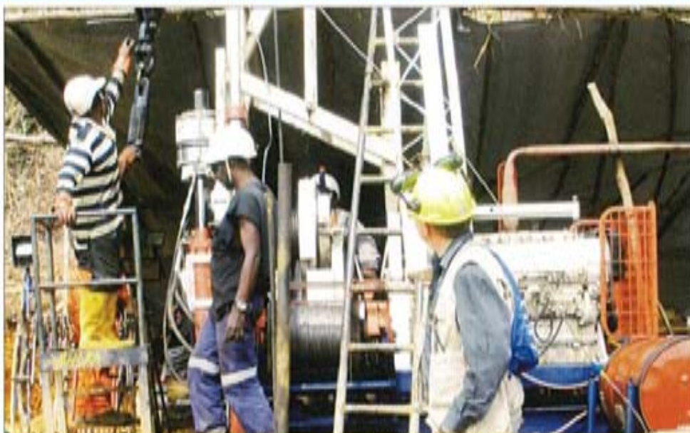
• Drilling at Mangla where workmen ensure all is safe before work begins.
